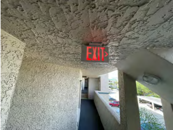
GENERAL VIEW OF EXIT LIGHTS
