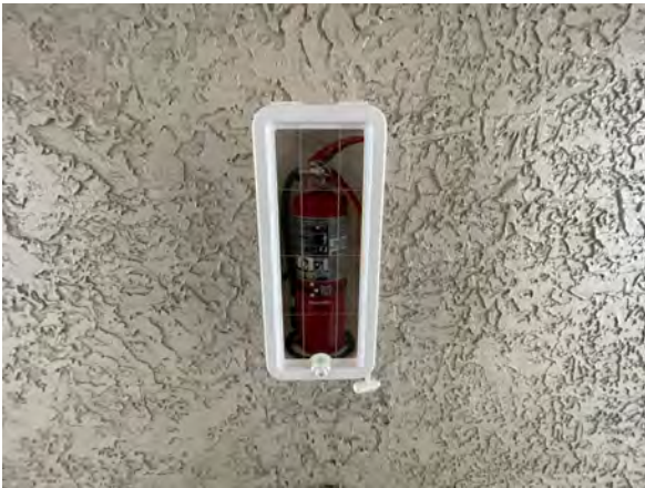
VIEW OF FIRE EXTINGUISHER
