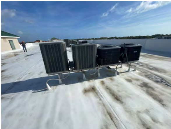
VIEW OF HVAC EQUIPMENT
