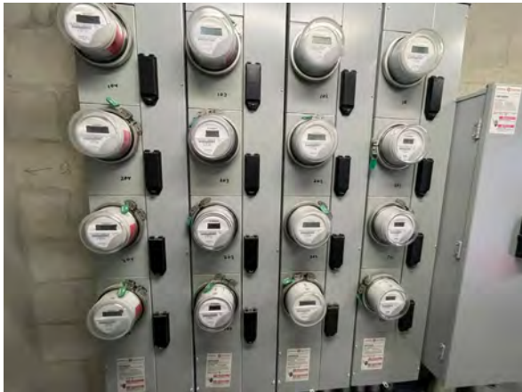
VIEW OF ELECTRICAL EQUIPMENT
