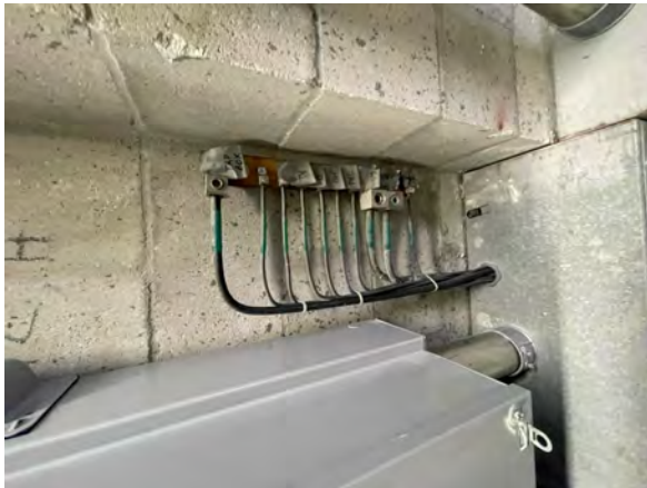
VIEW OF ELECTRICAL EQUIPMENT
