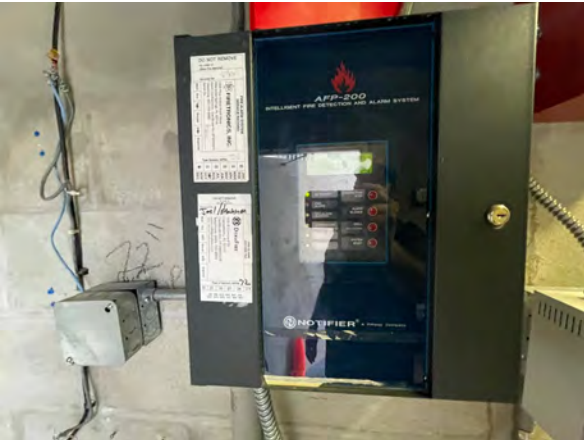
GENERAL VIEW OF FIRE ALARM PANEL
