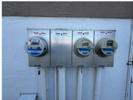
View of Electrical Equipment
