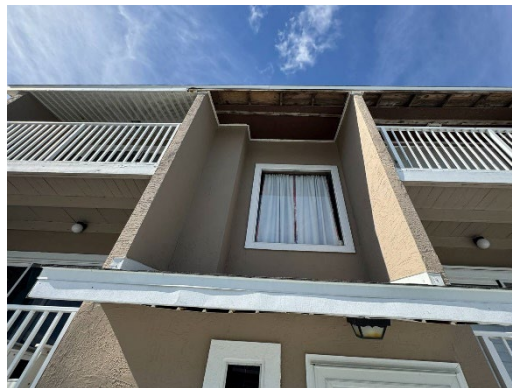
View of Damaged Soffit
