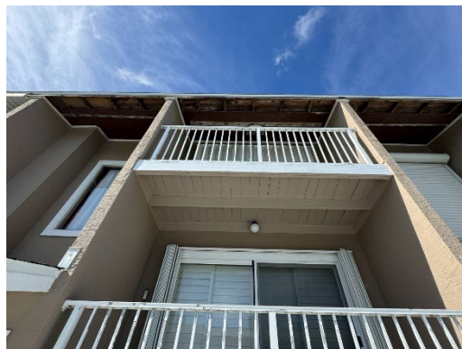
View of Damaged Soffit
