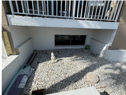
View of Minor Deterioration to Wood Balcony
