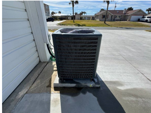
General View of HVAC Equipment
