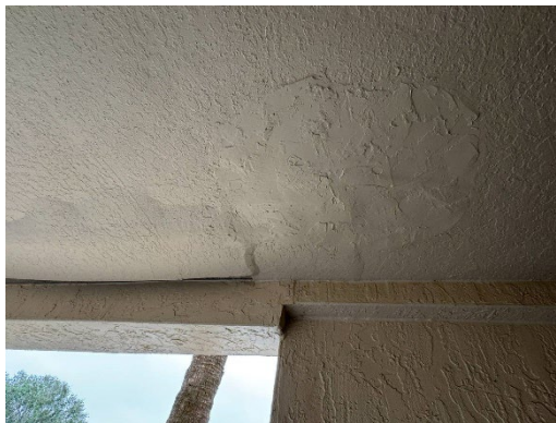
View of Bulging/Cracking in Stucco of previously repaired area on elevated walkway.
