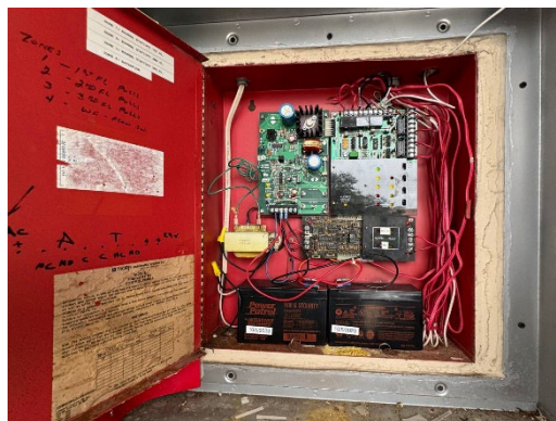
GENERAL VIEW OF FIRE ALARM PANEL
