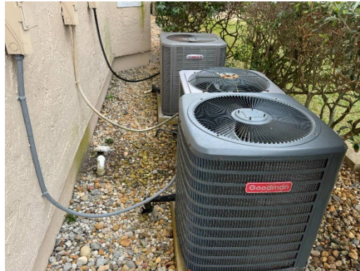
GENERAL VIEW OF HVAC EQUIPMENT
