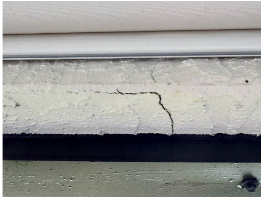
View of Stucco cracking at balcony beam.
