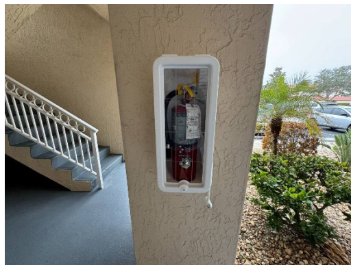
GENERAL VIEW OF FIRE EXTINGUISHER
