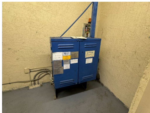
GENERAL VIEW OF ELEVATOR EQUIPMENT
