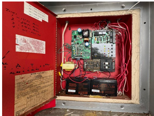
GENERAL VIEW OF FIRE ALARM PANEL
