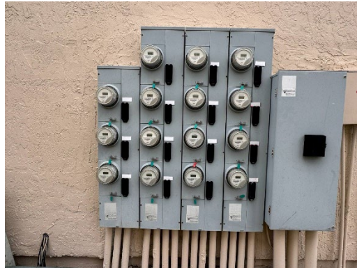
GENERAL VIEW OF ELECTRICAL EQUIPMENT
