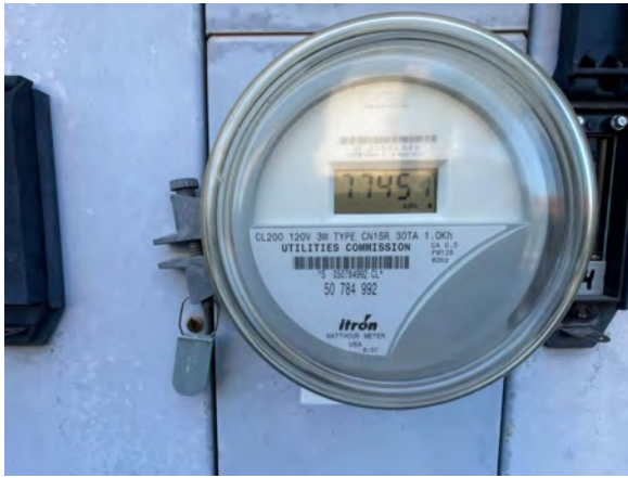
GENERAL VIEW OF ELECTRICAL EQUIPMENT
