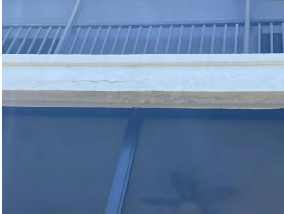
VIEW OF CRACKING STUCCO
