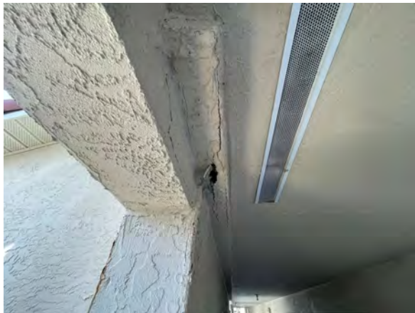
VIEW OF STUCCO CRACKING AND WATER INTRUSION
