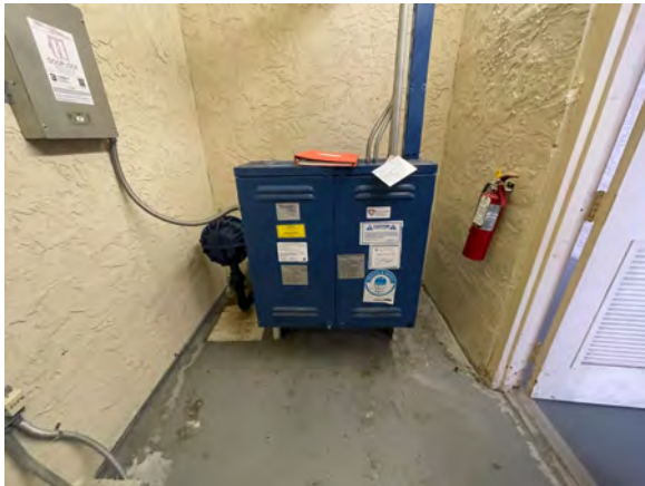
VIEW OF ELEVATOR EQUIPMENT
