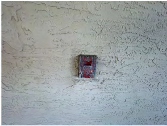
VIEW OF PULL STATION
