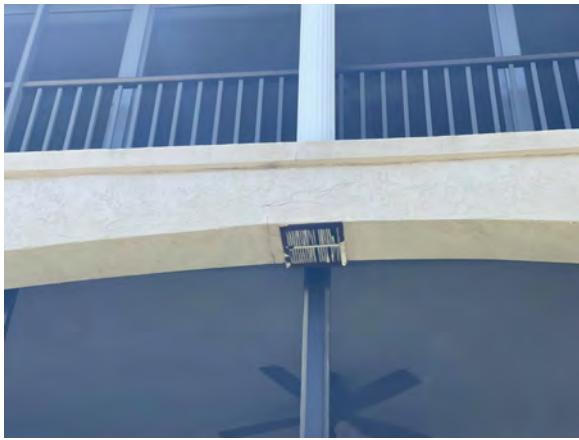
VIEW OF CRACKING STUCCO
