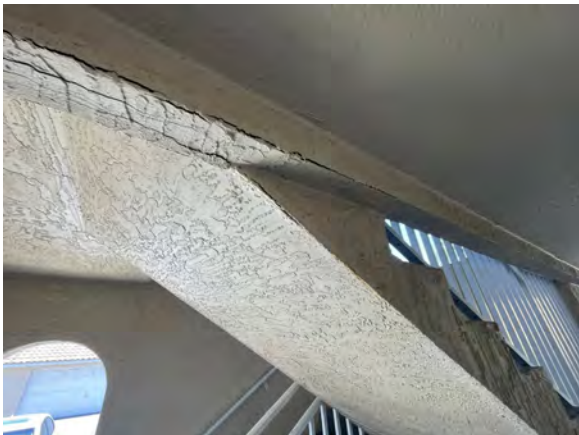
VIEW OF STUCCO CRACKING
