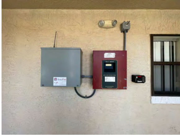
VIEW OF FIRE ALARM PANEL
