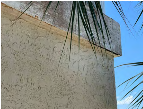
VIEW OF STUCCO CORNER BEAD DETERIORATION
