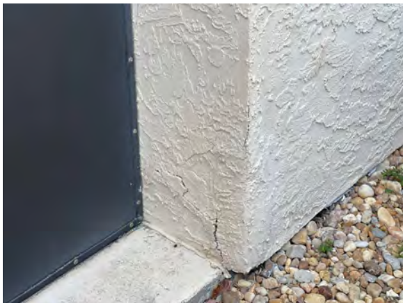
VIEW OF CRACKING STUCCO
