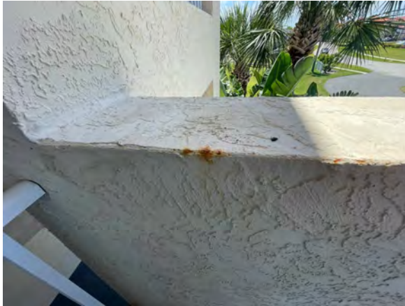
VIEW OF STUCCO CORNER BEAD DETERIORATION
