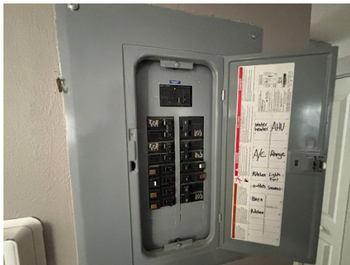
View of Electrical Equipment
