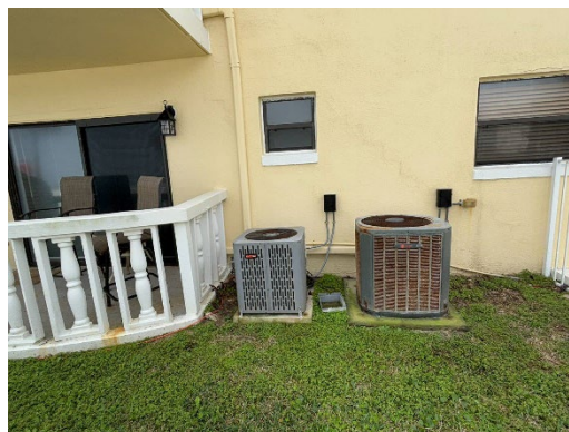
View of HVAC Equipment
