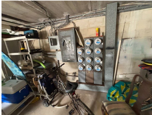
View of Electrical Equipment
